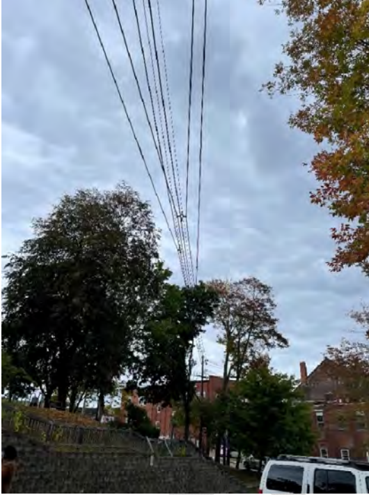
Photo 19 – Overhead hydroelectric lines
