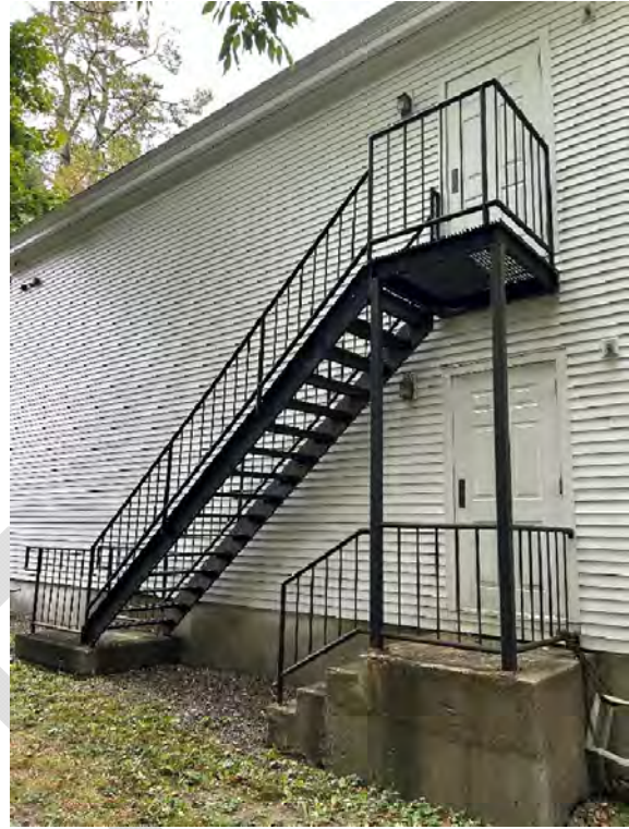
Exterior Egress Stairs Exposed to Weather
