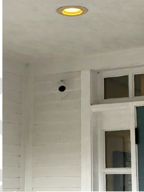
Exterior Security Camera
