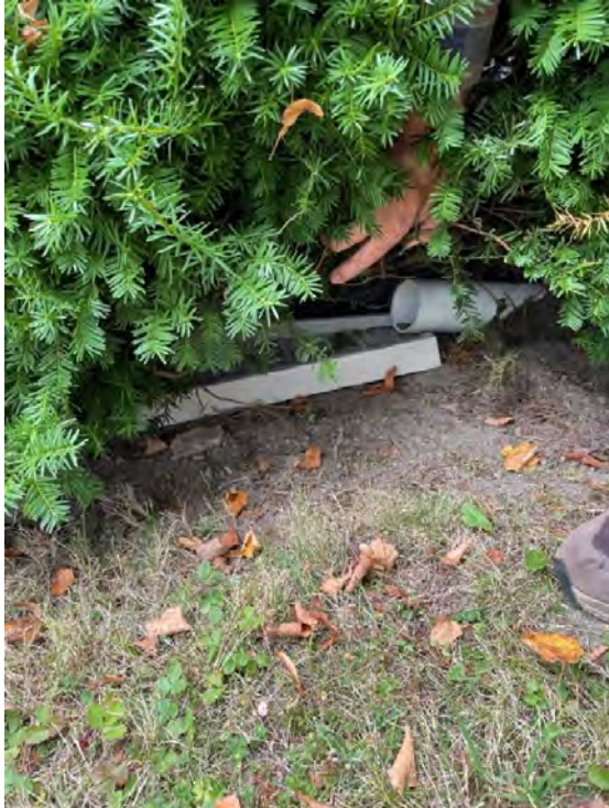
Photo 15 – Basement sump pump outfall, typ of two
