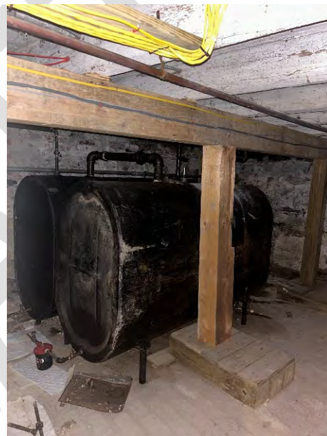
Existing Oil Tanks
