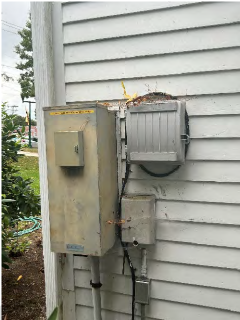
Exterior Electric Service
