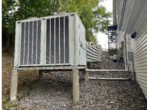
North Condensing Units
