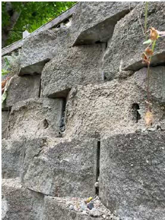
Photo 23 – Close up of deteriorated block facing
