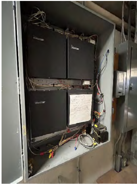
Existing Control Panel
