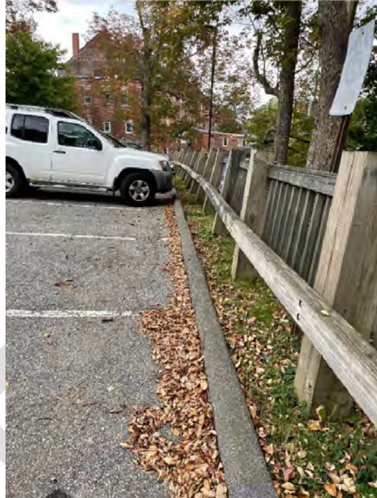
Photo 26 – Tilting timber guardrail
