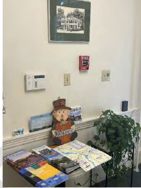
Fire Alarm Pull Station
