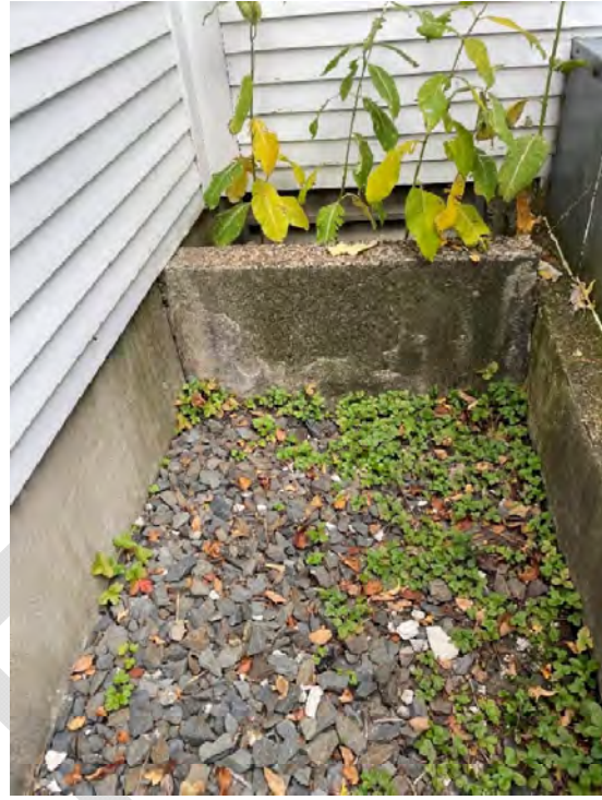
Photo 16 – Eastern well for fresh air intake, drainage issues
