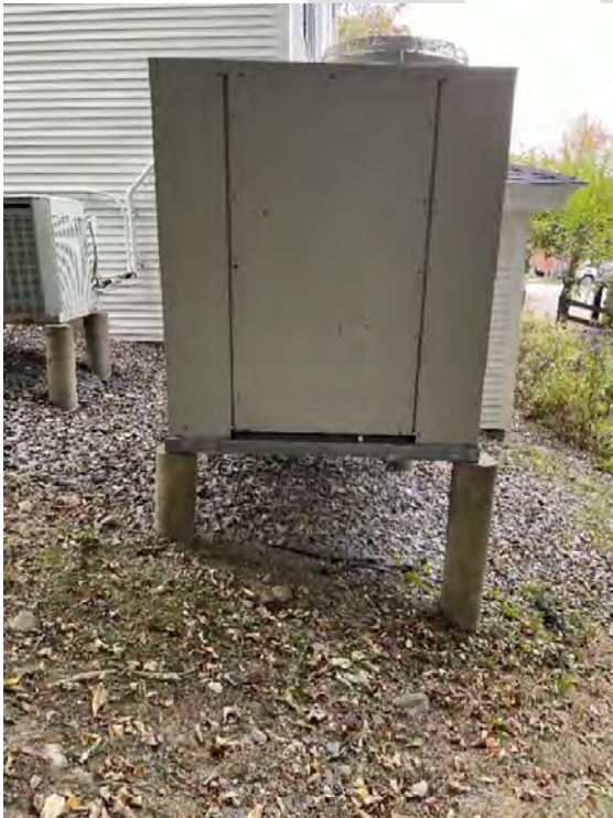
Photo 7 – Tilting sonotube HVAC supports (see mechanical section)
