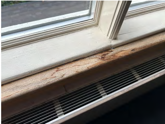
Water-Stained Sill at the New Addition
