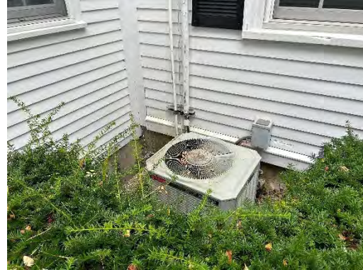
Central Condensing Unit
