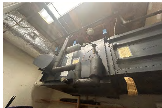
Basement Air Handler
