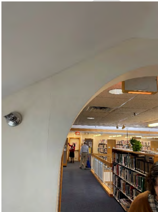
Photo 17 – Connector to addition, drywall cracks
