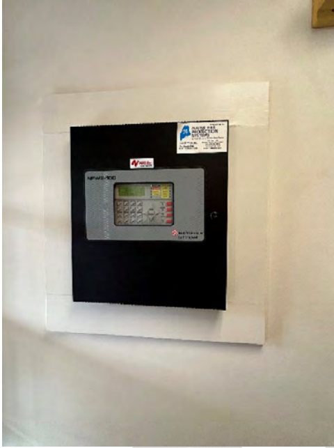
Fire Alarm Control Panel
