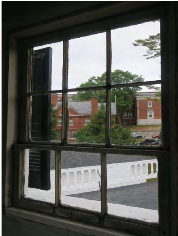
Single-Pane Window at the Cupola Showing a combination of old and new windows
