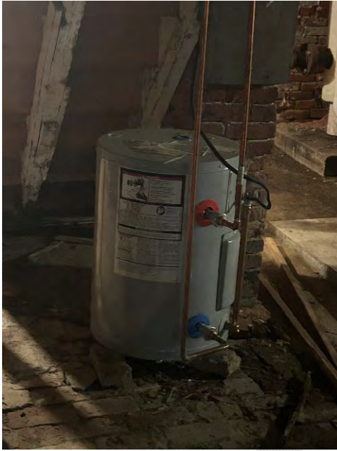
Electric Water Heater
