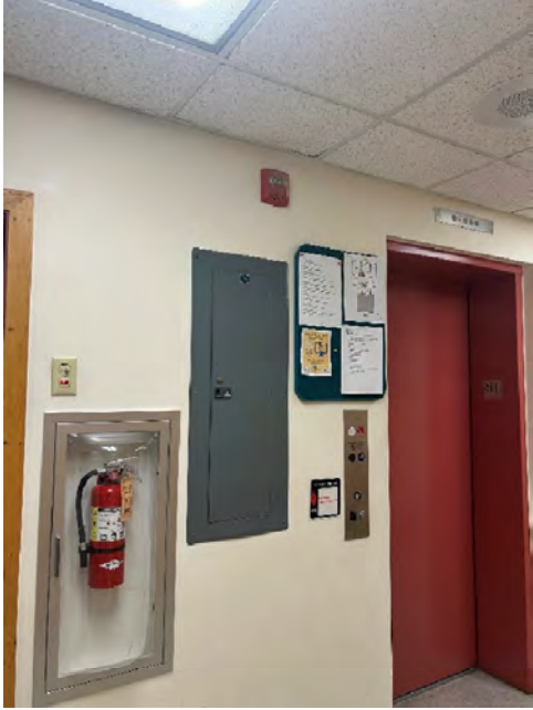
Fire Alarm & Strobe
