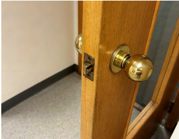
Non-Accessible Hardware at the New Addition
