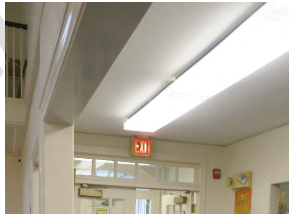
First Floor Hall Lighting at the Tisdale House
