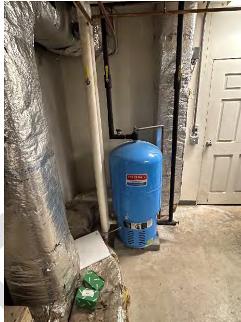
Existing Boiler Mate
