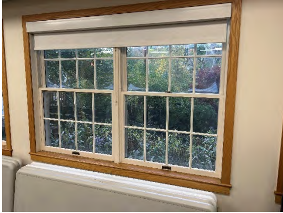
Fogged Glass at the New Addition
