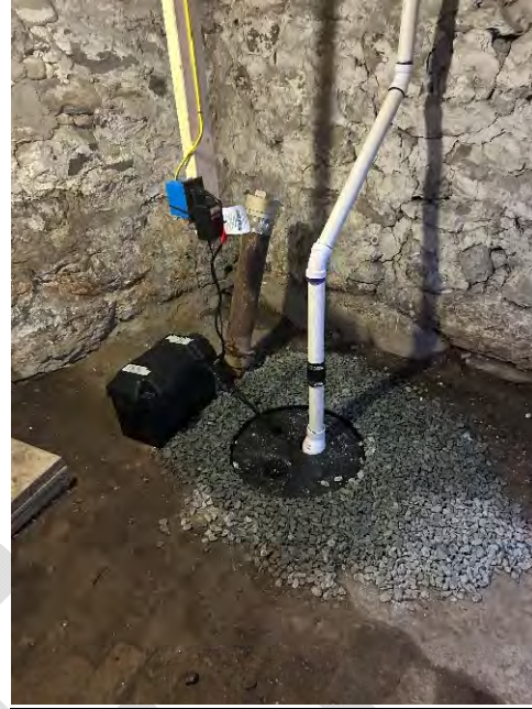
NW Sump Pump
