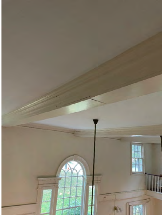
Photo 15 – Original ceiling, cracked trim
