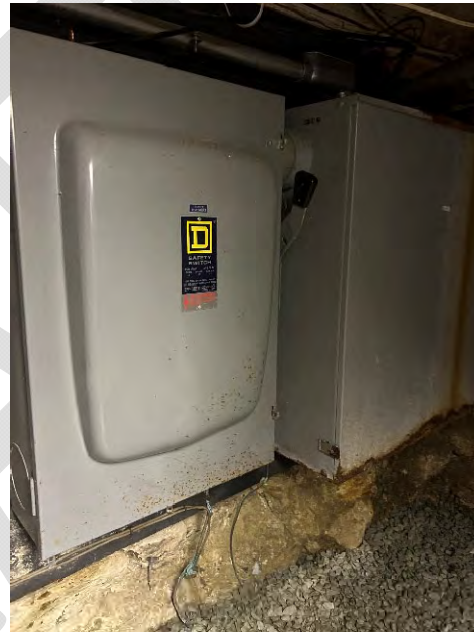
Interior Electric Panels
