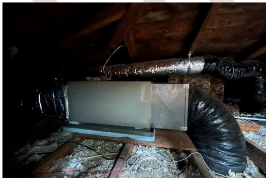
Attic Air Handler
