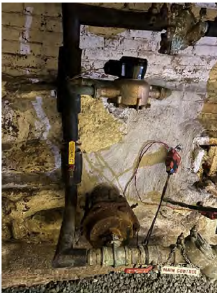
Domestic Water Service
