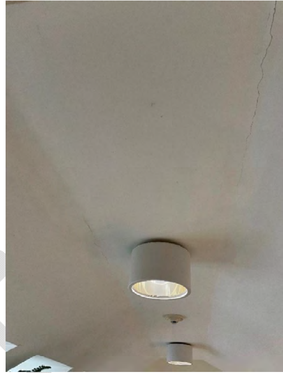
Photo 16 – Connector to addition, drywall cracks in ceiling
