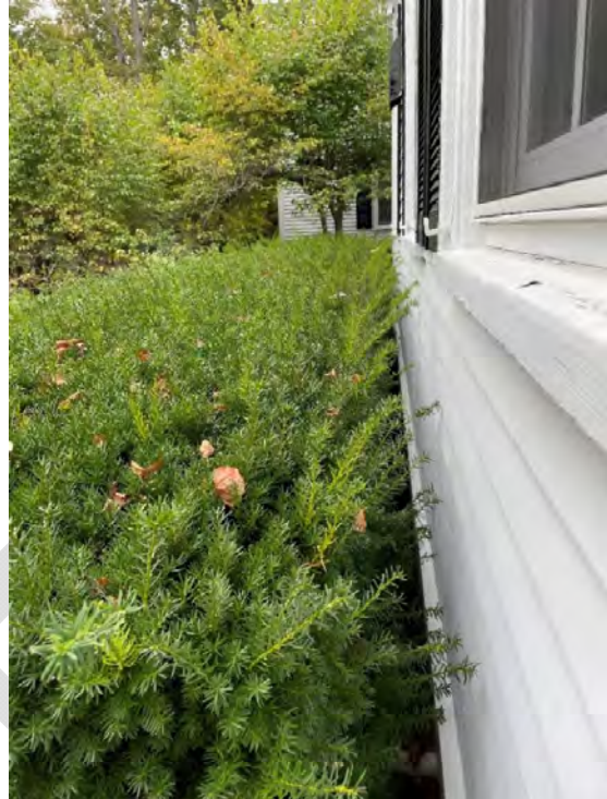
Photo 30 – Vegetation against building
