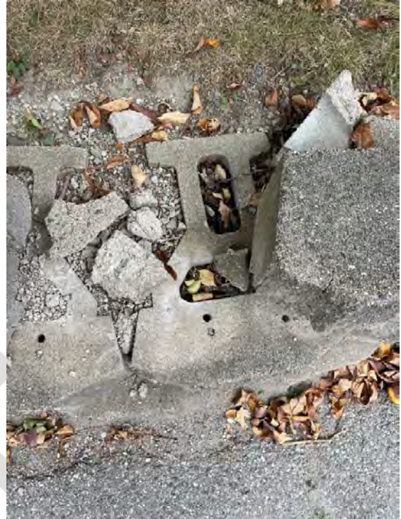
Photo 22 – Close up of deteriorated block caps
